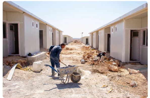
In 2022, the humanitarian community has started to implement its dignified shelters action plan in north-west Syria. So far, more than 2500 dignified shelters have been implemented and more than 19,700 are in progress. (Photo: BINAA for Development)
