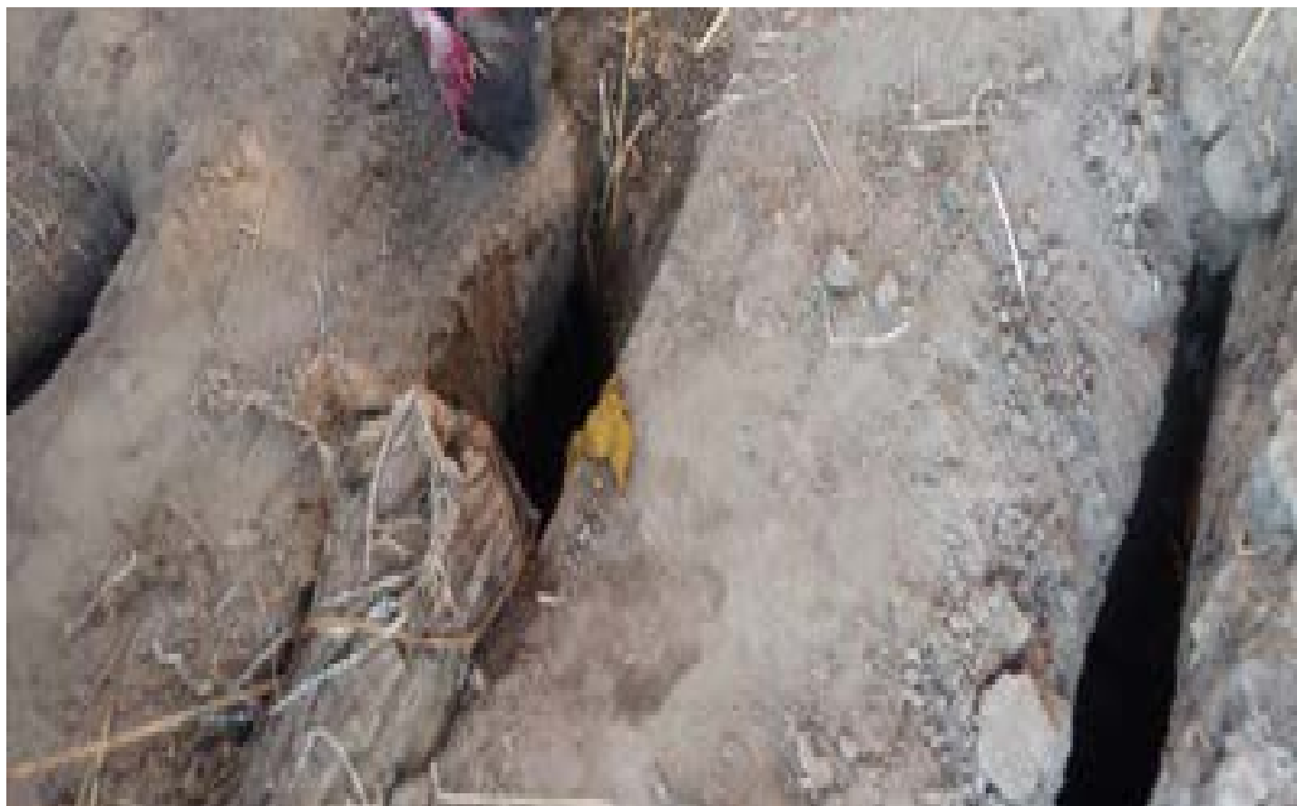
Figure 2. Unimproved latrine at a household of one of the confirmed case of cholera. Dust, open floor with faeces on it
