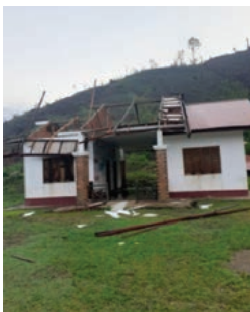
FIG. 27. Roofing destroyed by an extreme weather event
