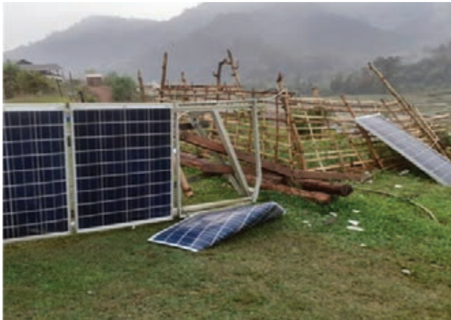
FIG. 28. Solar panels destroyed by an extreme weather event
