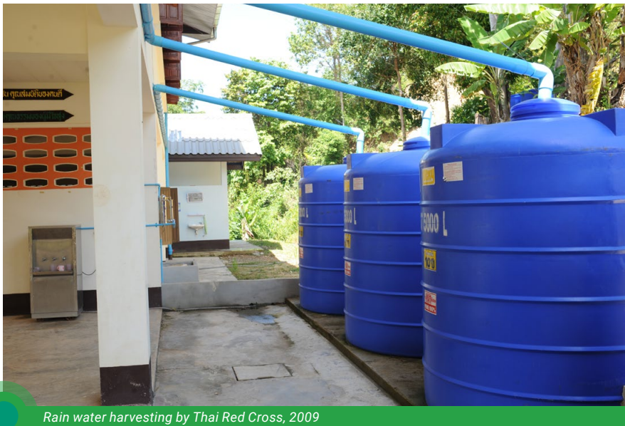
Rain water harvesting by Thai Red Cross, 2009
