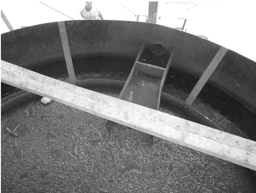
Photo 7.2 Arrangement for scum removal, Sittwe hopper-bottomed tank
