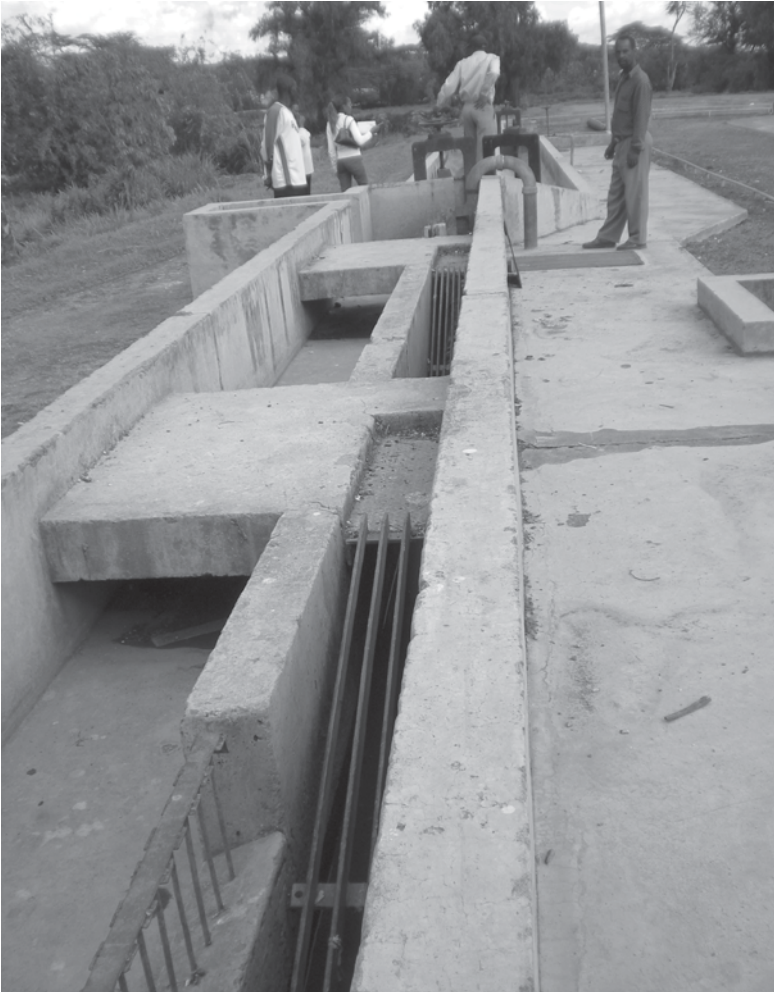
Photo 5.3 Inclined screen with operator access
