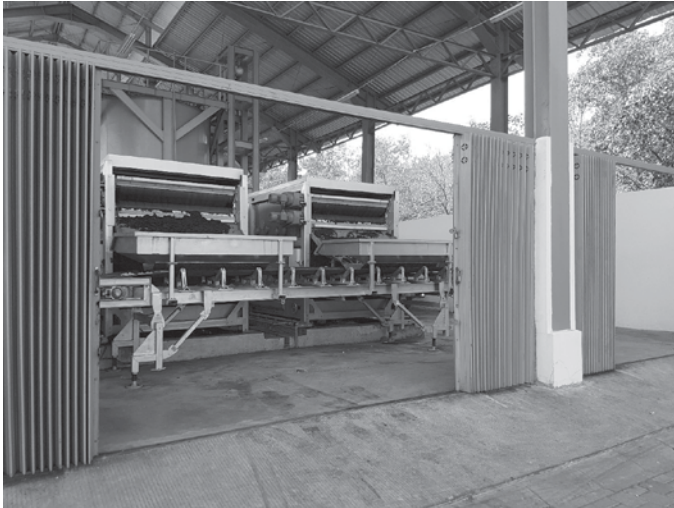
Photo 7.4 Belt filter press at Duri Suwung Septage Treatment Plant, Denpasar, Indonesia Source: Chengyan Zhang of Stantec
