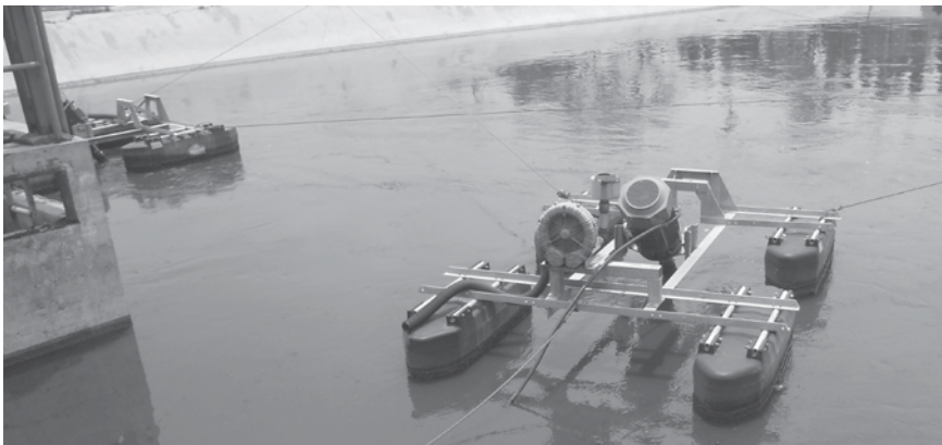
Photo 8.2 High-speed surface aerator at Duri Kosambi, Jakarta
