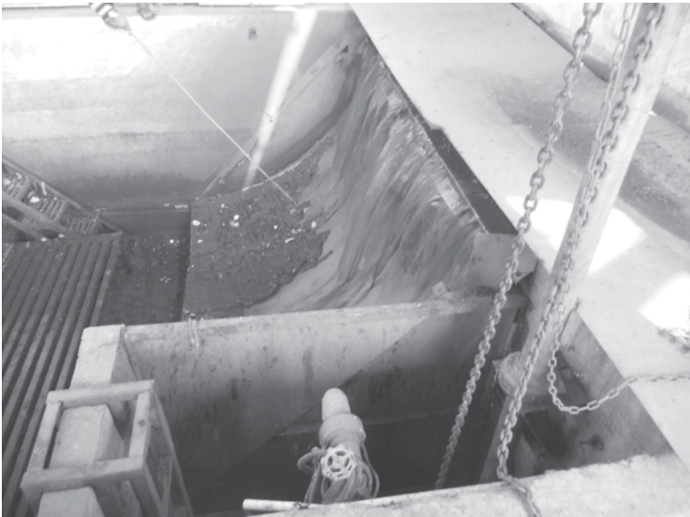
Photo 6.7 Run-down screen at Pula Gebang septage treatment plant
