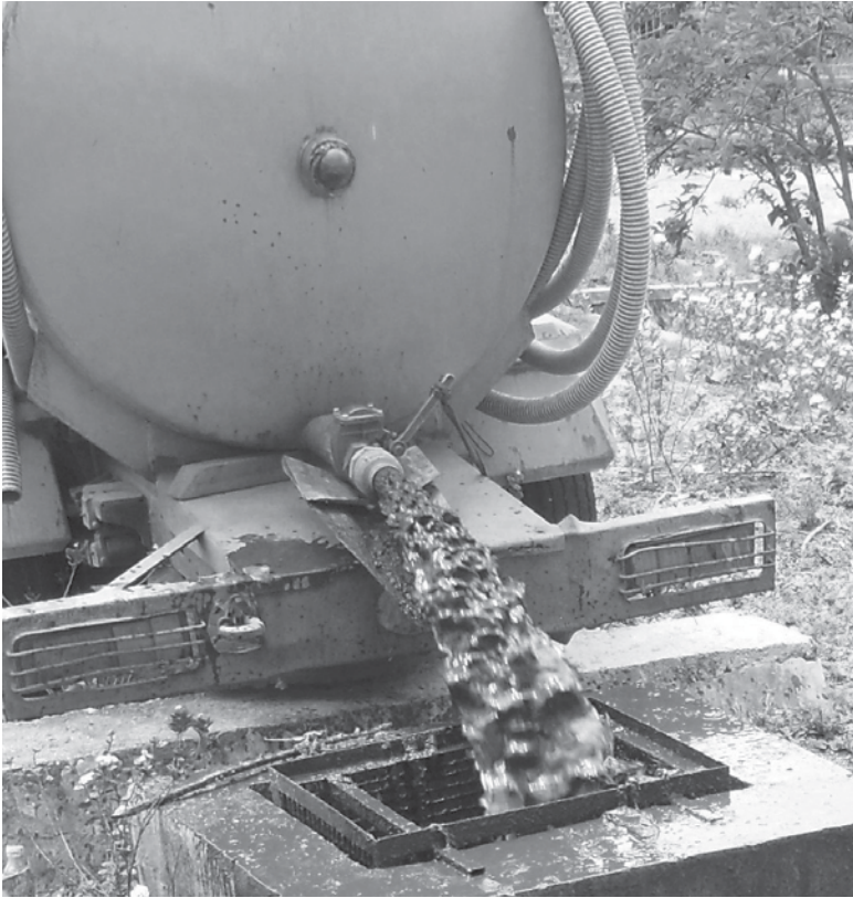
Photo 6.1 Direct discharge to an Imhoff tank: an unsatisfactory arrangement resulting in spillage
