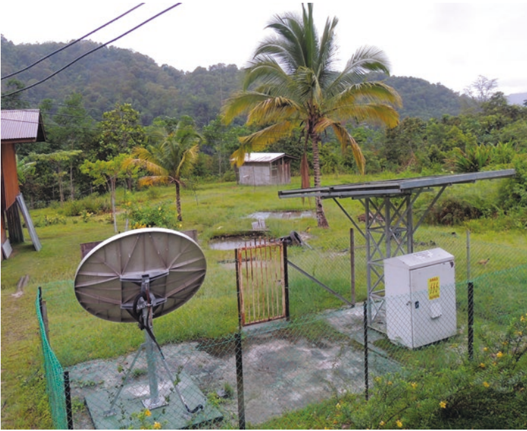
Fig. 26.4 A village micro-grid energy and telecommunications system in the Crocker Highlands of Sabah, Malaysian Borneo. The system serves a community of 200 and provides household energy services, telecommunications, and a satellite communications (dish shown), water pumping for fish ponds (seen in the center), and refrigeration. The supply includes micro-hydropower and solar generation (one small panel is shown here; others are distributed on building rooftops). (Photo credit: Daniel M. Kammen)
