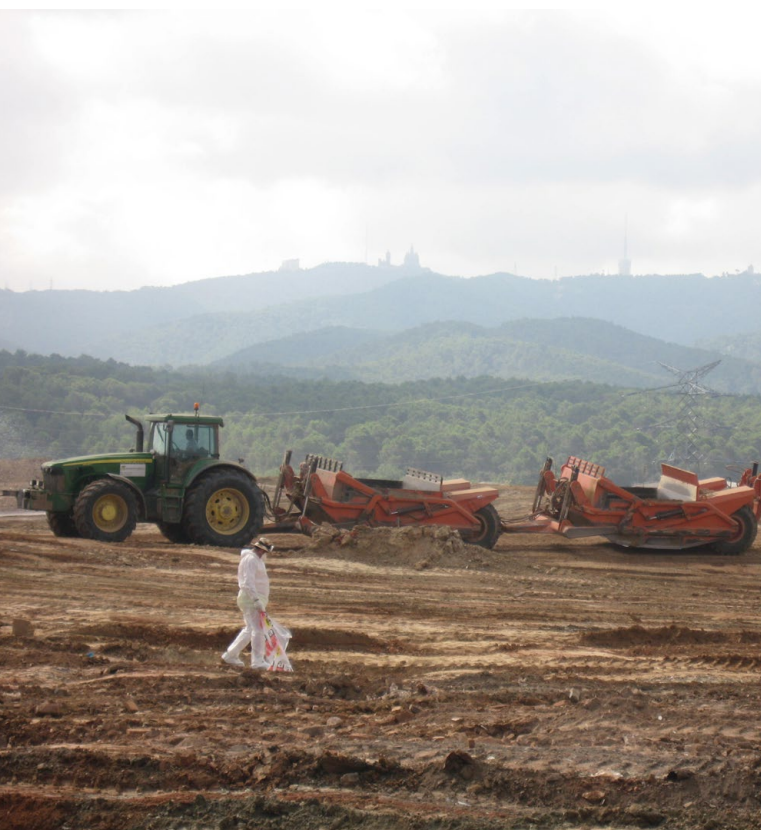
Remediation work and capping to prevent asbestos exposure at Parc de l'Alba, Spain © Parc de l'Alba
