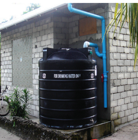
Rain water harvesting
