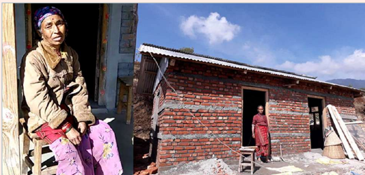
Image 28: Eet Maya in front of her under-construction home. Source: HRRP District Team, 2020
