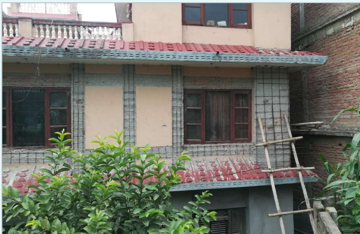
Image 22: Mesh being laid out for external jacketing of Kanchan Thapa's house. Source: HRRP District Team, 2020
