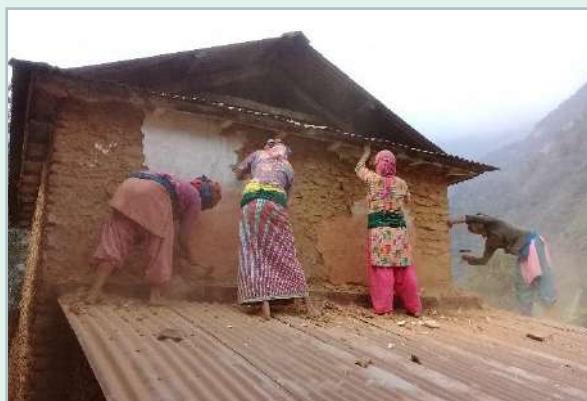
Image 18: The old layer of plastering being chipped off for retrofitting. Source: HRRP District Team, 2019
