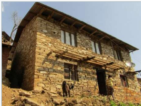
Image 2: House of Suresh Shrestha which was partially damaged by the earthquake. Source: NSET
