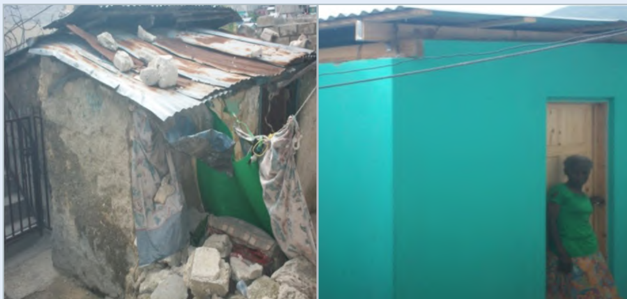
Image 31: Left: Before repair and retrofit; Right: After repair and retrofit. Source: CRS Haiti
