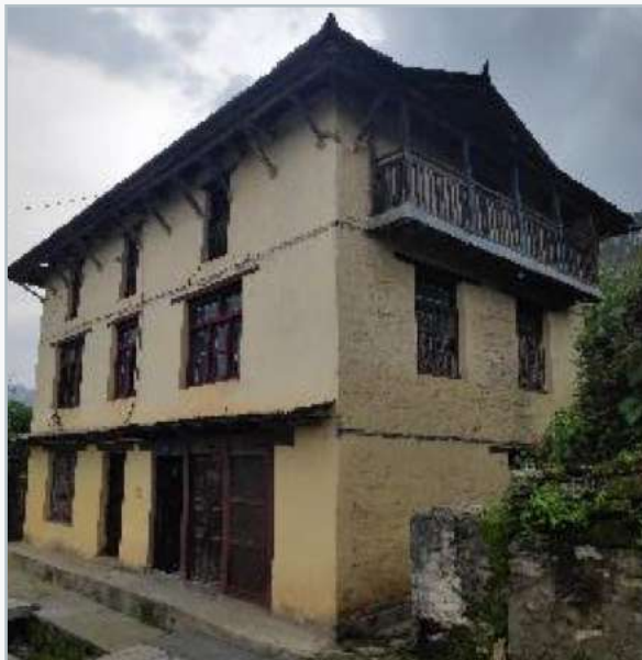
Image 4: Partially damaged traditional house of Ananda Bahadur Shrestha which lies in Dwalkha traditional settlement area. Source: NSET
