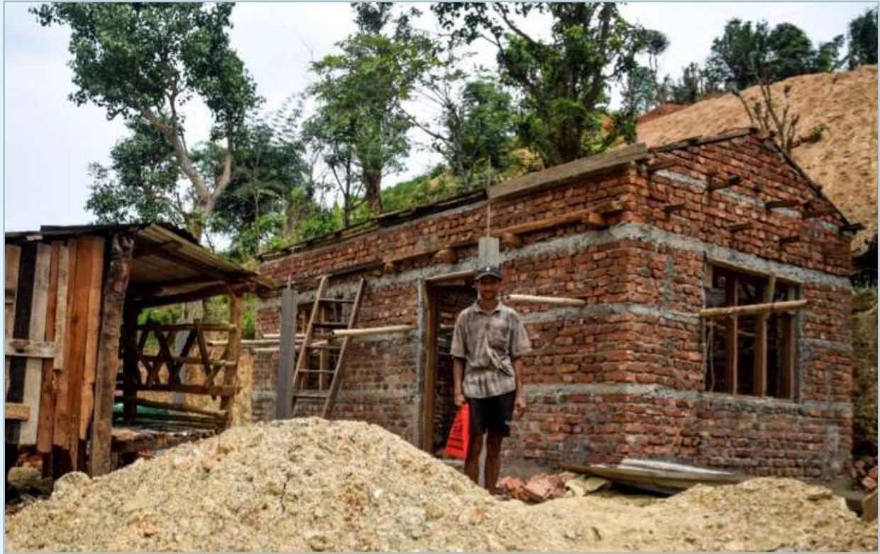
Image 11: Mr. Arjun Sunar in front of his house under reconstruction. Source: UNDP, Nepal
