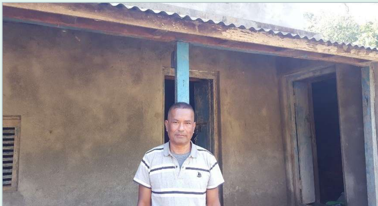
Image 20: Mr. Hari Bahadur Thapa in front of his retrofitted house. Source: HRRP District Team, 2019
