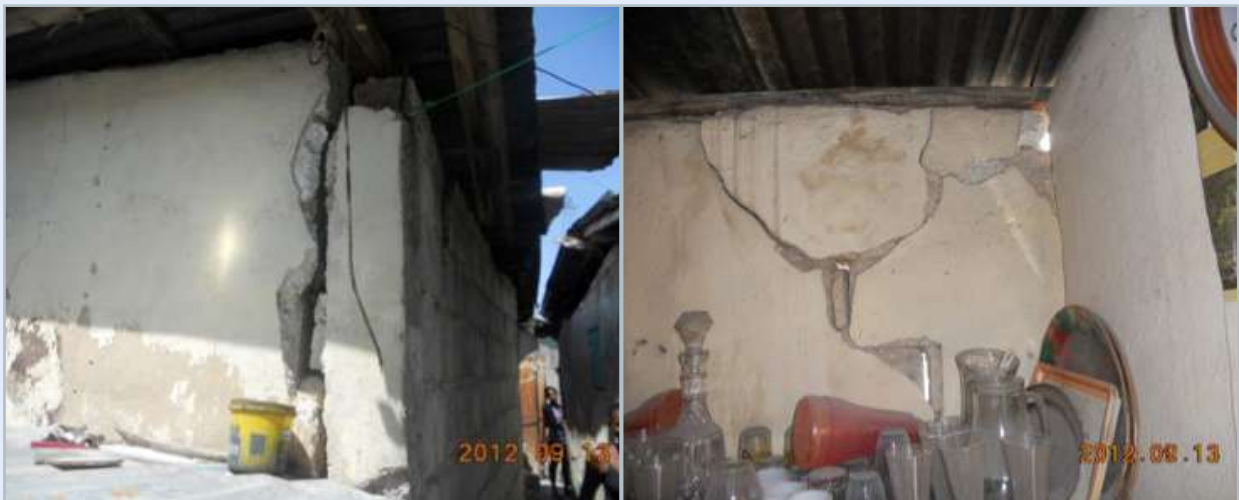
Image 30: Photos showing the condition of houses after the earthquake. Source: CRS Haiti
