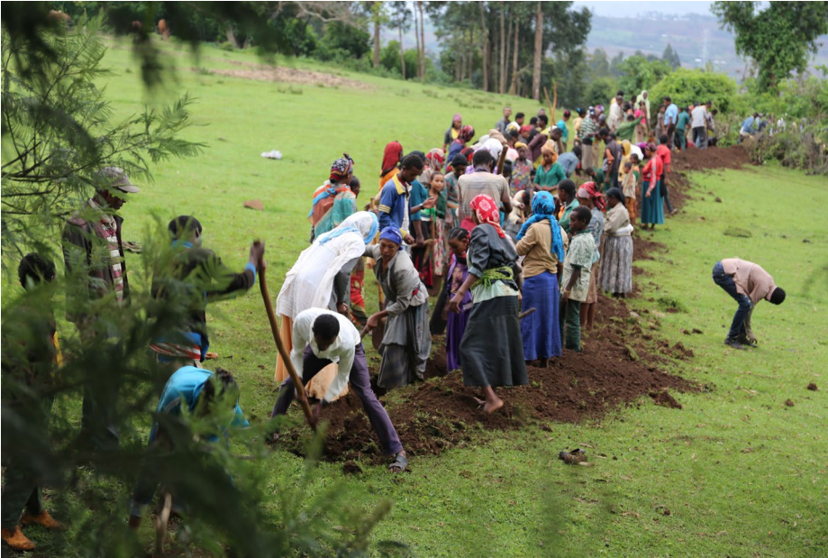
Figure 5.2 Community members provide their labour to dig a trench for their new water supply.
