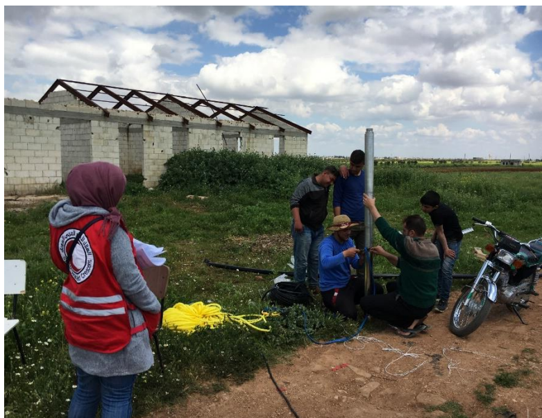
SARC staff supervising the water pump installation work in Homs. Photo: SARC.
