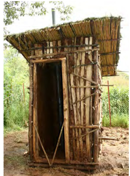
VIP latrine made from mud and wattle.
