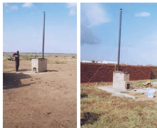
Figure 15 - Photos of double-chamber incinerator
