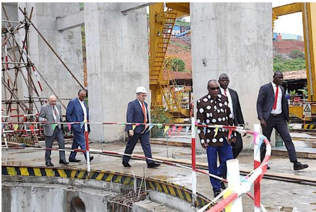
President Alpha Condé visits the construction site of the Souapiti dam on June 12, 2019. The Guinean government hopes that the 450-megawatt dam will increase access to electricity in a country in dire need of more reliable power. © 2019 Guinean President's Office
