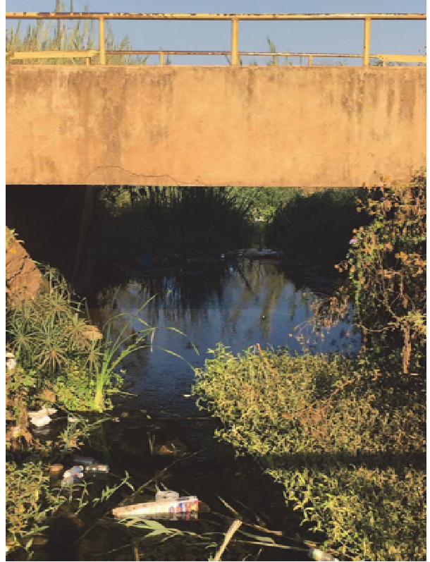
The former mine canal, pictured here, which discharged mine waste when the mine was still operational, annually becomes clogged with weeds and debris. It then floods during the rainy season, contaminating adjacent neighborhoods with lead.
