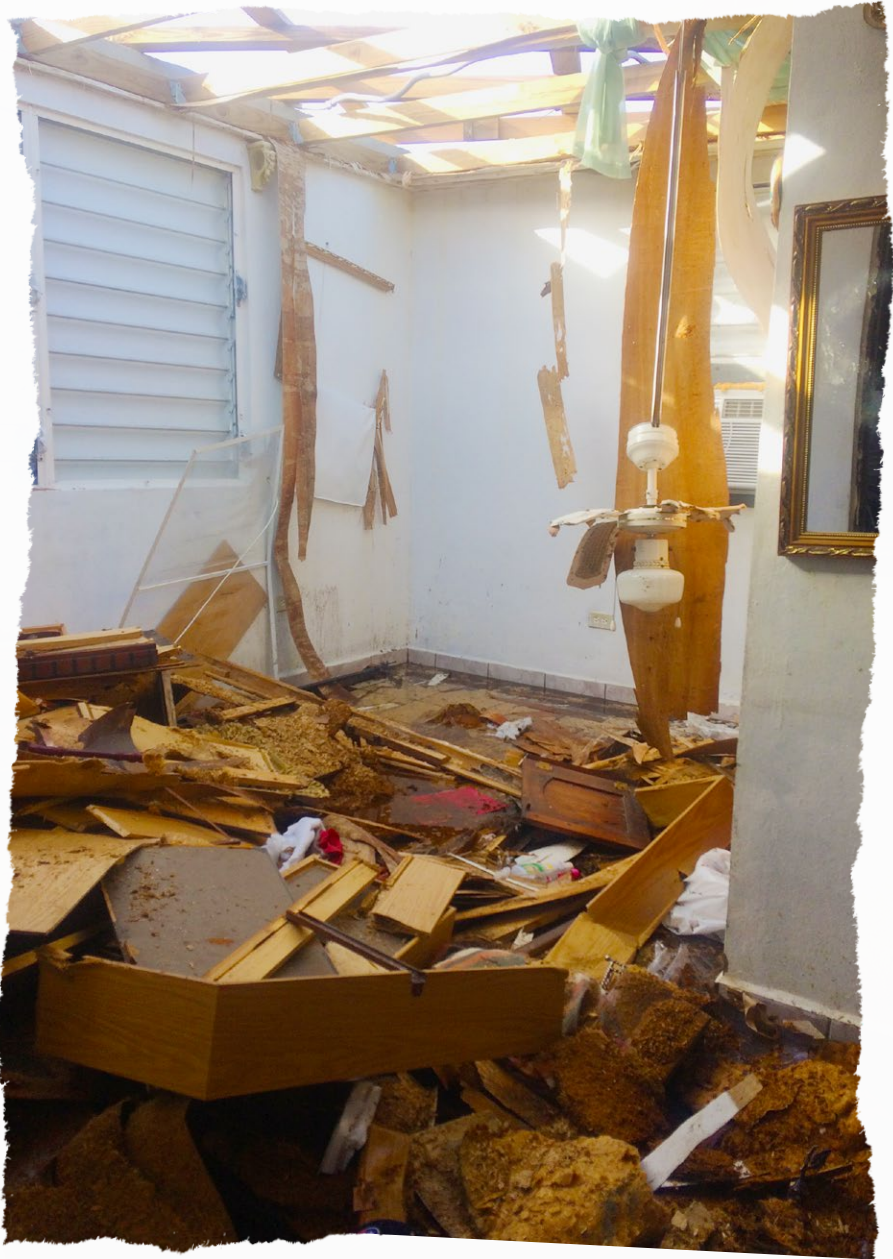
Interior of a damaged house in Ingenio, Puerto Rico Source: Dr. Gemma Sou, October 2018.
