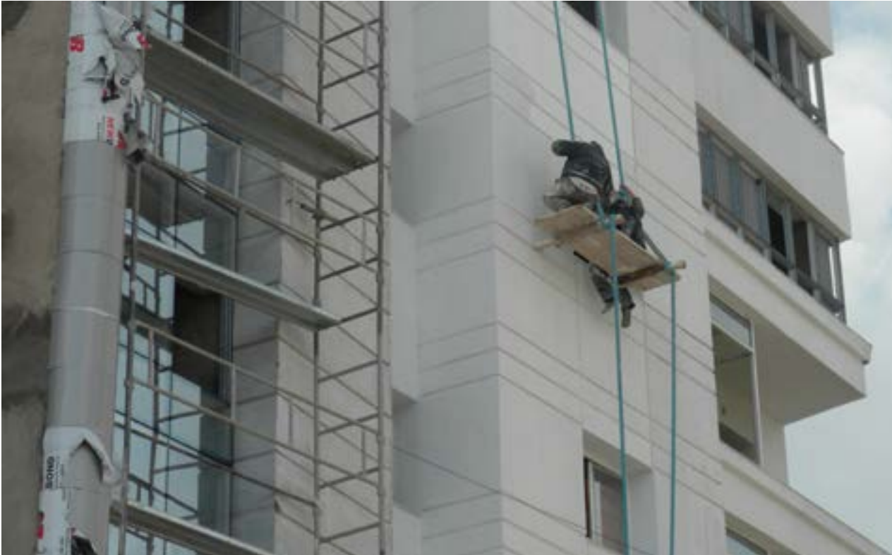
Construction workers work on a building in Tunisia with little safety protection. (Credit: Khaled Abelmoumen)
