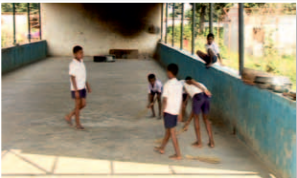
School without boundary wall and inadequate infrastructure 24
