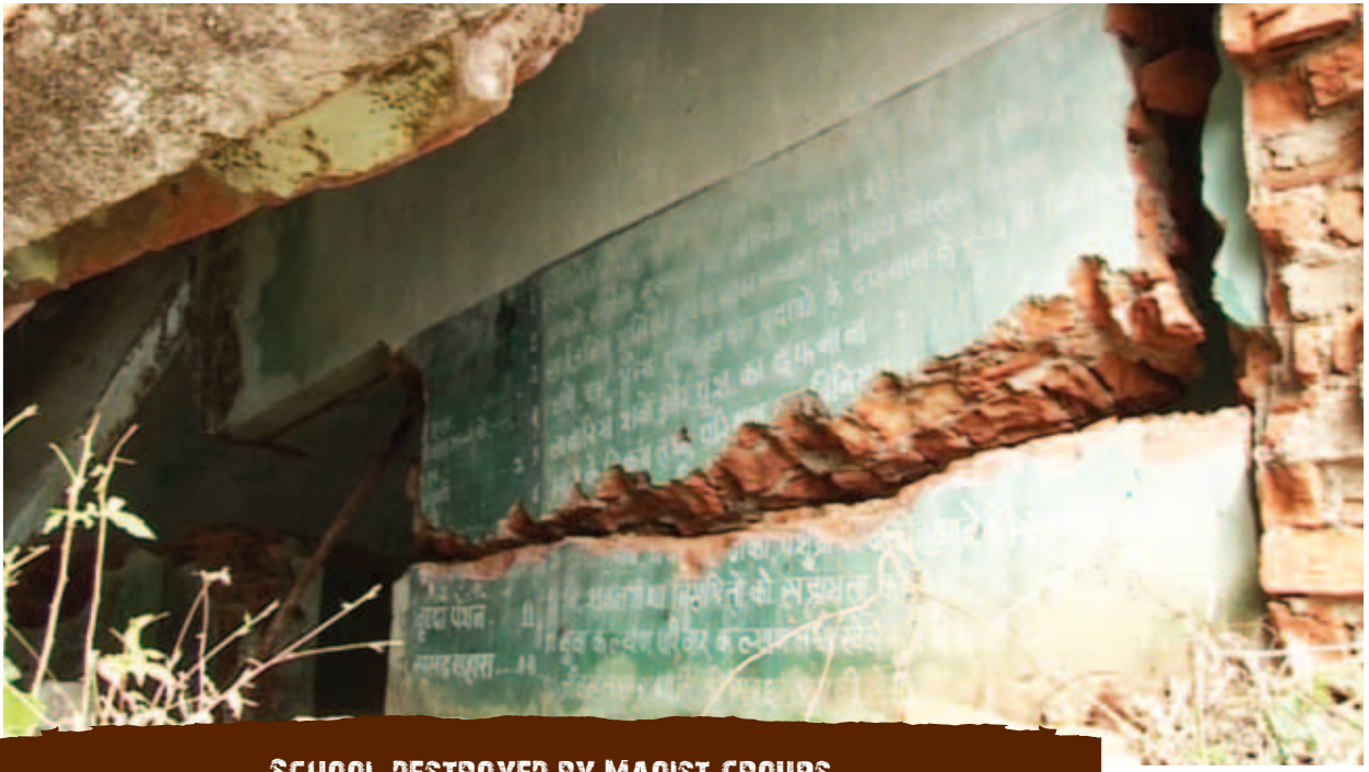
SCHOOL DESTROYED BY MAOIST GROUPS
