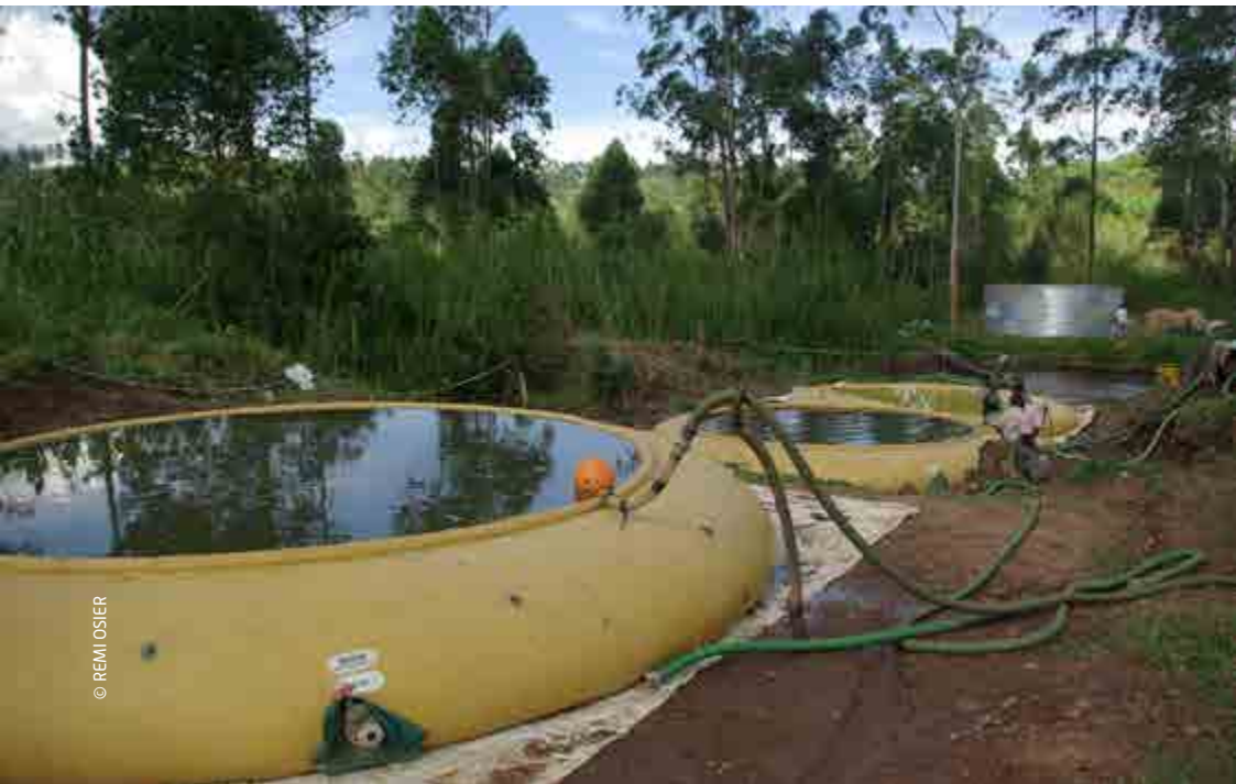
Photo 2 - Onion tanks set up in a drinking water treatment plant
