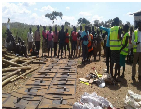
Distribution of latrine construction material and digging kits. Picture by Paul Semakula
