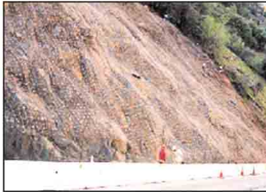
Source: www.engineering4theworld.org/LAP Figure 3-4: Net used to prevent stone fall on a roadway
