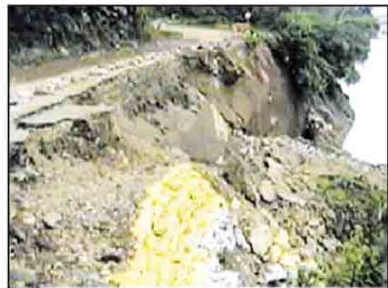
Photo@ U Kyaw Tun Figure 2.5 Road Slide due to Heavy Rain(Kalewa-Kale Road)
