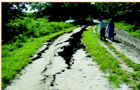
Fissures formed during 2003 Taungdwingyi Earthquake, central Myanmar
