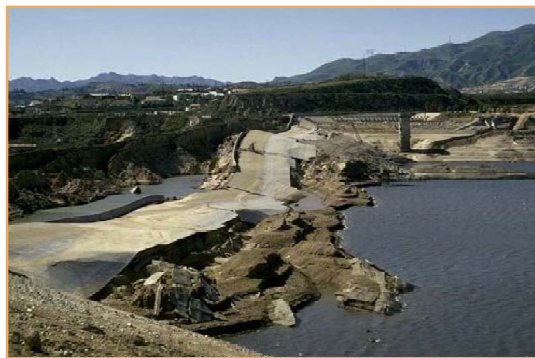
Lower Van Norman Dam experienced widespread liquefaction and major slope failures during the 1971 San Fernando Earthquake
