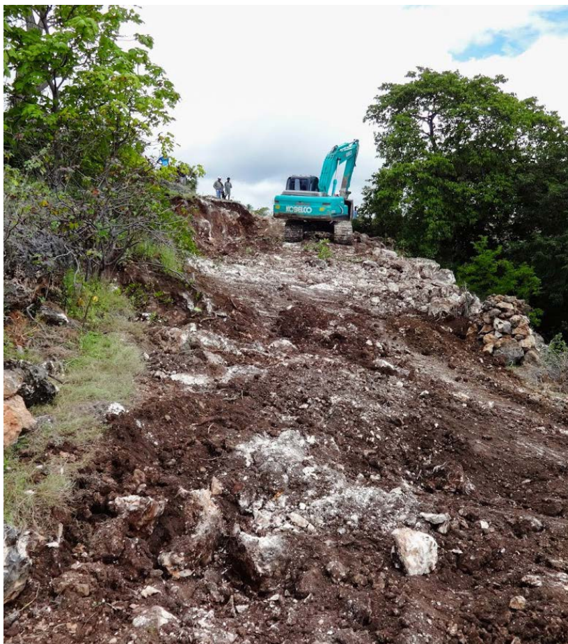
Photo 11: Poor Road Conditions in Rural Areas of Timor-Leste
