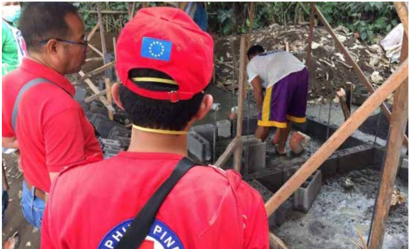
Photo 8: Philippine Red Cross Building Latrines for Disaster Victims
