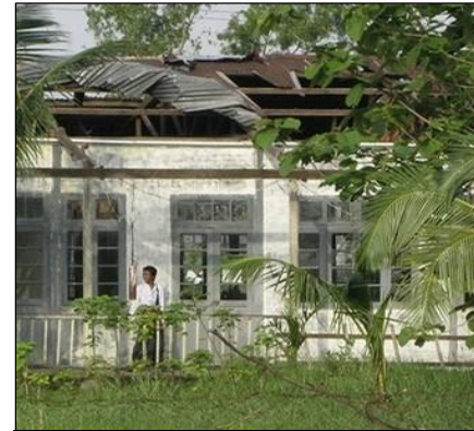
A young school boy walking along the verandah of a damaged school in Thuwana, Yangon.
