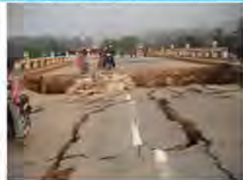
Figure 1.4.3 Damaged road and bridge structure (Source: http://globalvoicesonline.org/2011/03/25/myanmar-photos-of-earthquake-disaster/economic )
