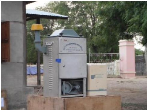
Ambient Air Quality Monitoring
