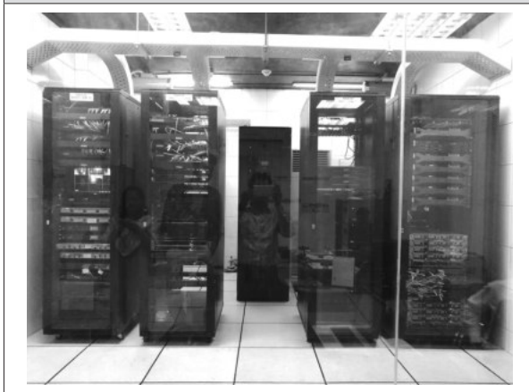
Figure 6.17. Picture of Data Center, MIS-DGHS
