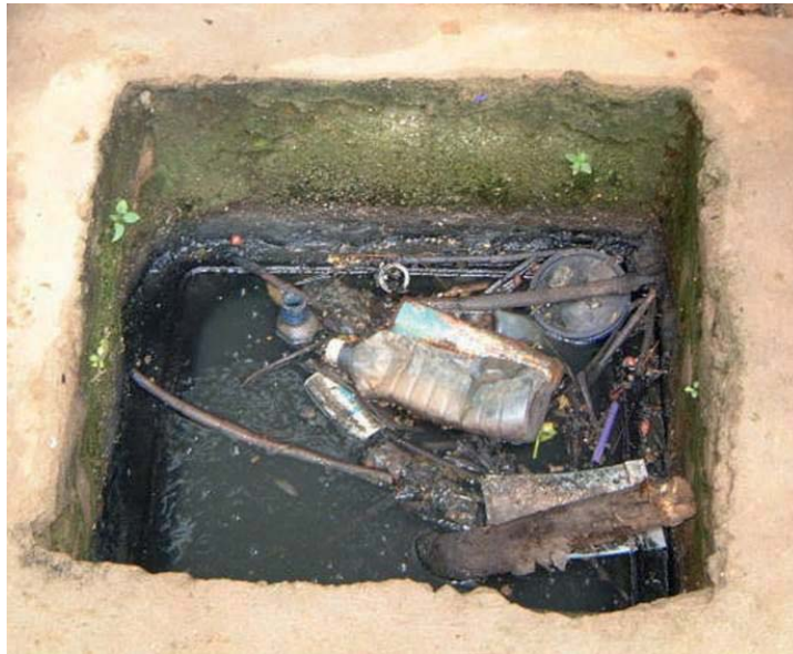
Fig. 27. Drains are excellent breeding sites for culicines and should be cleaned, treated or made inaccessible to vectors (photo courtesy of S. Lindsay)
