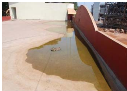
Figure 47. Blocked terrace with water © Ashwani Kumar
