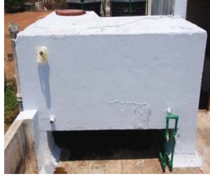
Figure 43. Vent pipe of an overhead tank covered with nylon mesh © Ashwani Kumar
