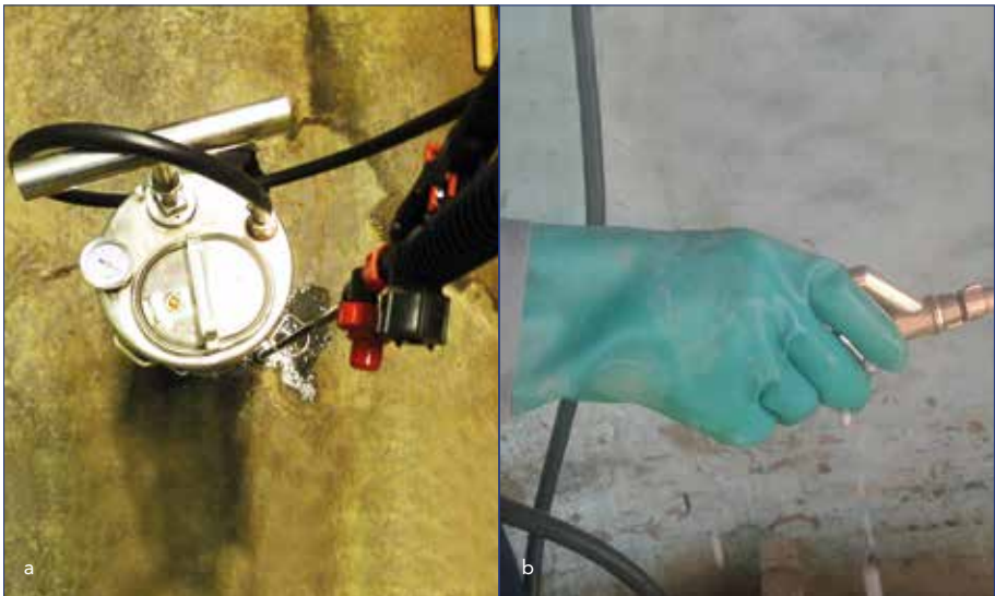
Figure 6. Equipment showing leakage from the trigger valve connection
