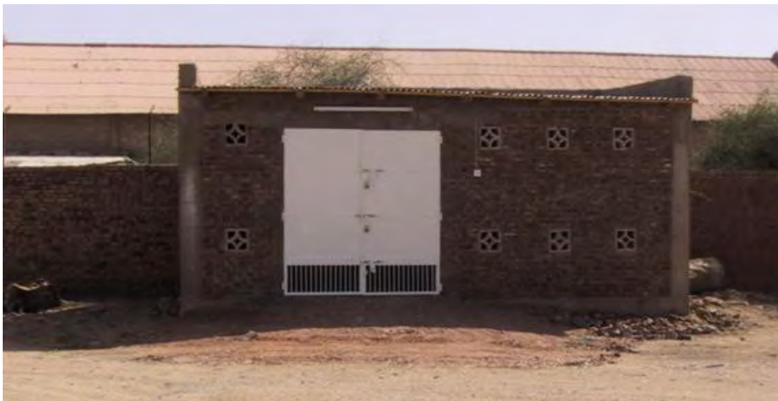
Figure 17.20 Dedicated dangerous goods store
