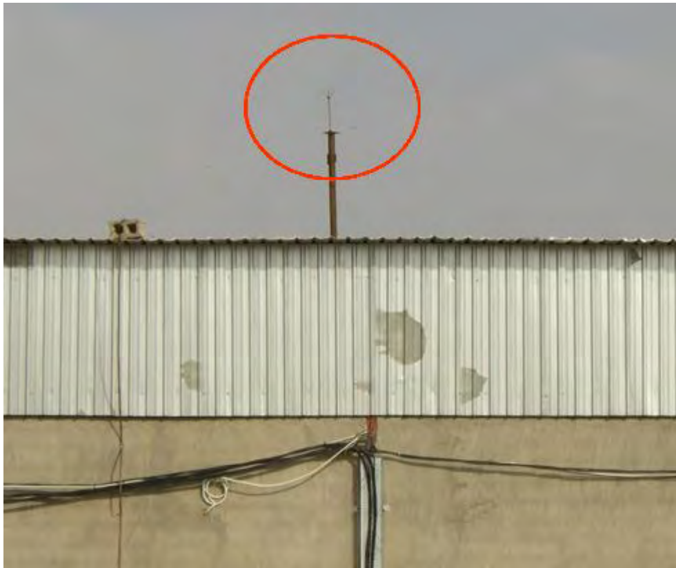
Figure 5.3 Arrestor (lightening protection)
