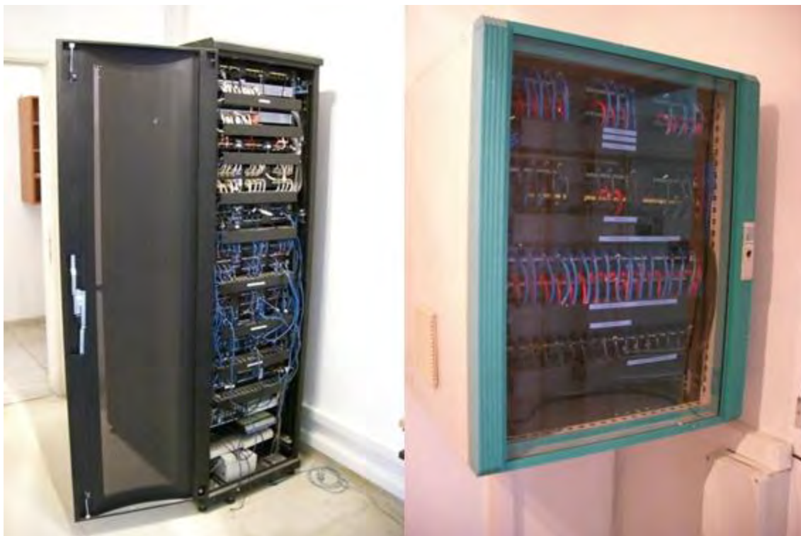
Figure 4.1 Computer network server
