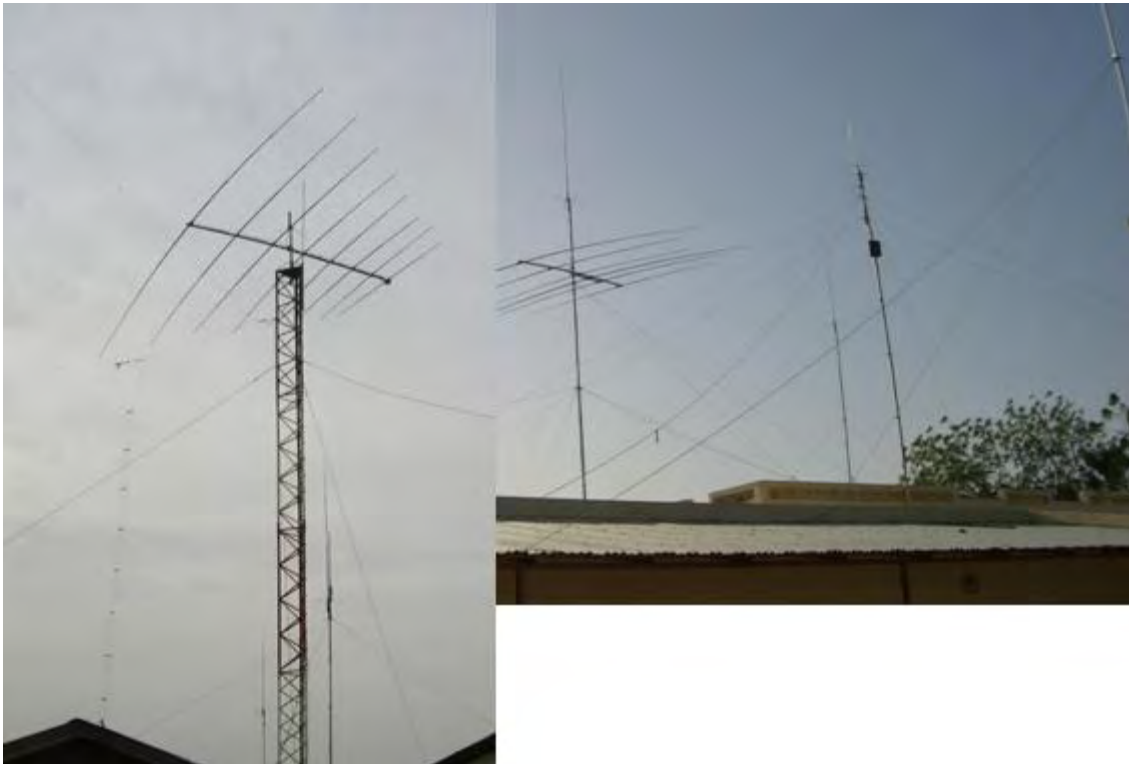
Figure 5.2 Example of radio aerials
