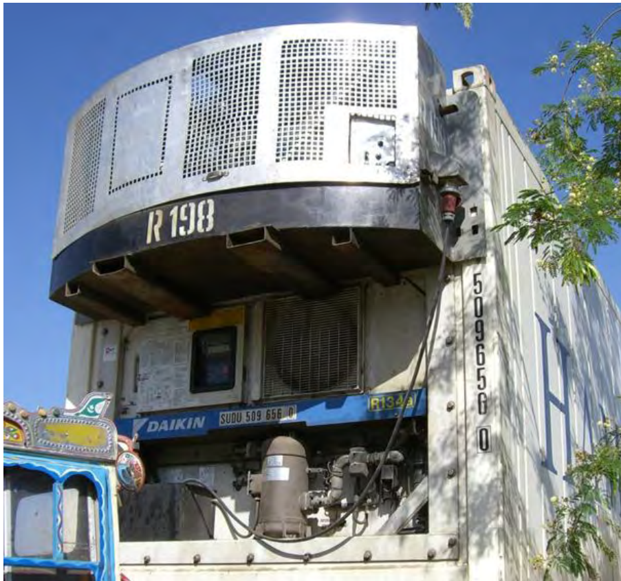
Figure 23.8 Cooling unit on refrigerated truck
