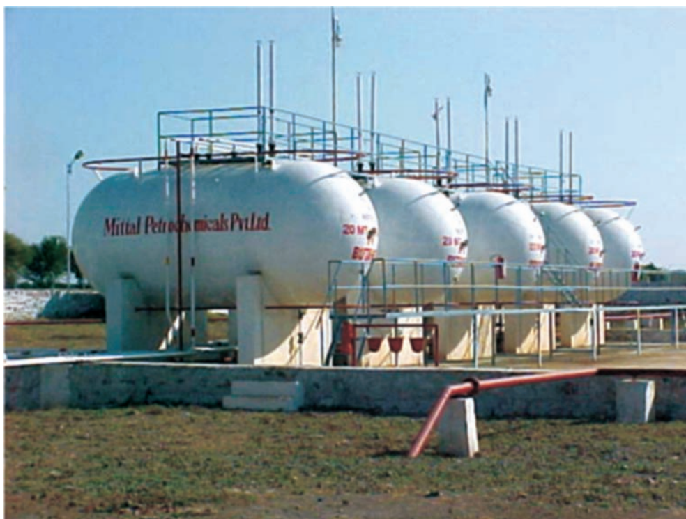
Figure 23: Chemical Storage units
