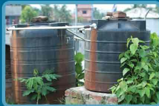
If the surrounding of roof tank remains untidy
