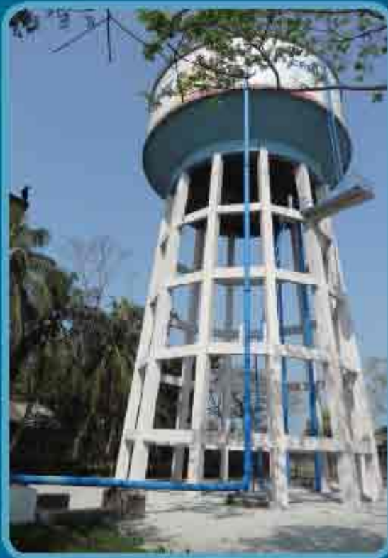
Piped water supply system
