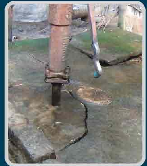
Sanitary seal does not exist at the base of tube well
