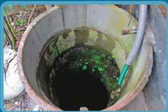
If inner portion of the underground reservoir remains unclean
