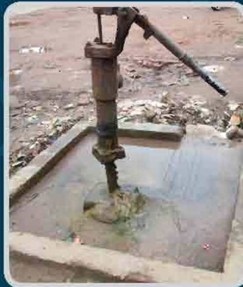
The platform is unclean, lichen grown up, garbage exists in the surroundings and water used by the drain doesn't drain out properly
