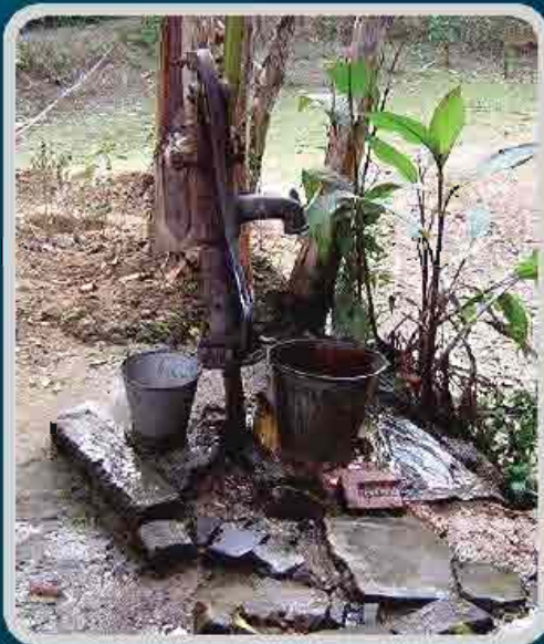
There is no platform or the platform is broken
