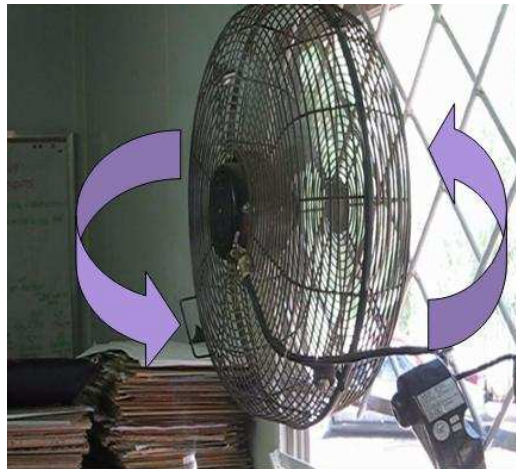
Figure 2: Examples of poorly-installed exhaust fan in an open window space, with “short-circuiting” of air-flow. In this installation, the fan adds little to ventilation; removal of the fan was recommended, as natural ventilation was adequate.
