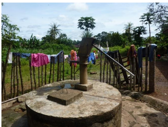
Figure 50: Baoma station water pump, Bo District
