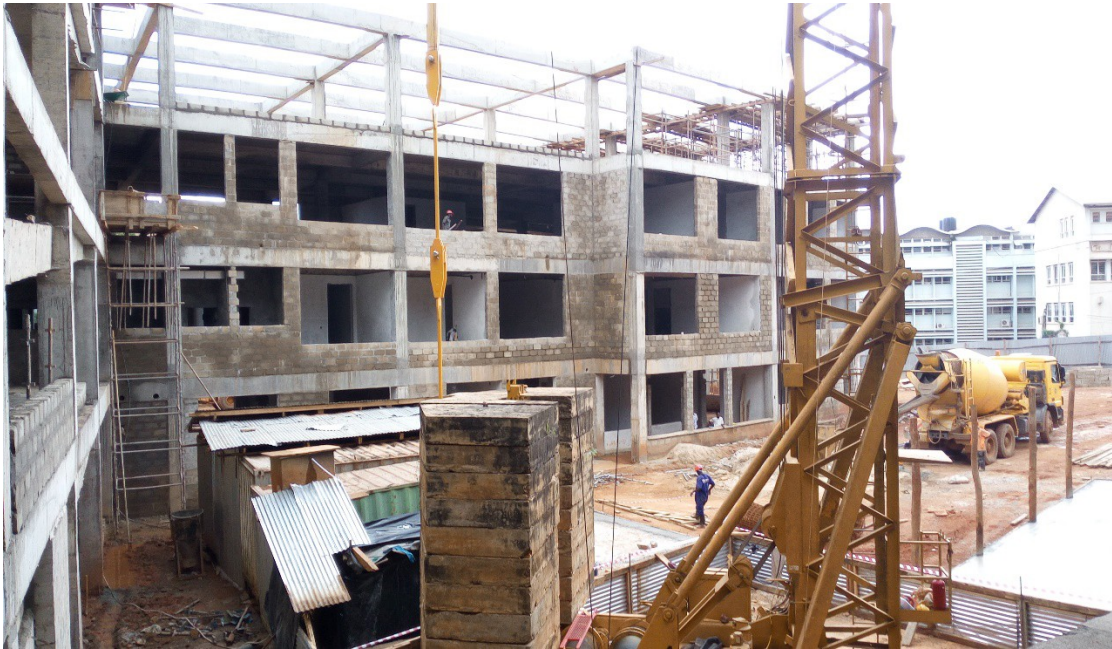
Works to one of the wings/ Blocks to house the ICU, Laboratory and Workshop now at level 4, in progress
