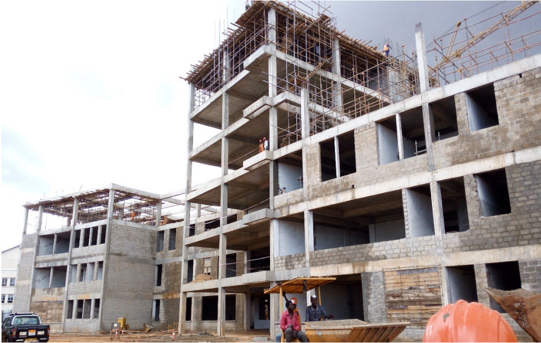
Structural frame of the Healthcare Unit built up to level 6 (at the main entrance)
