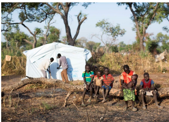
Sudanese refugees outside their new home in Ajuong Thok camp, South Sudan, as staff from UNHCR partner Danish Refugee Council fix the exterior walls. All new arrivals in Ajuong Thok are provided land and shelter materials to build their new home. UNHCR / Rocco Nuri
