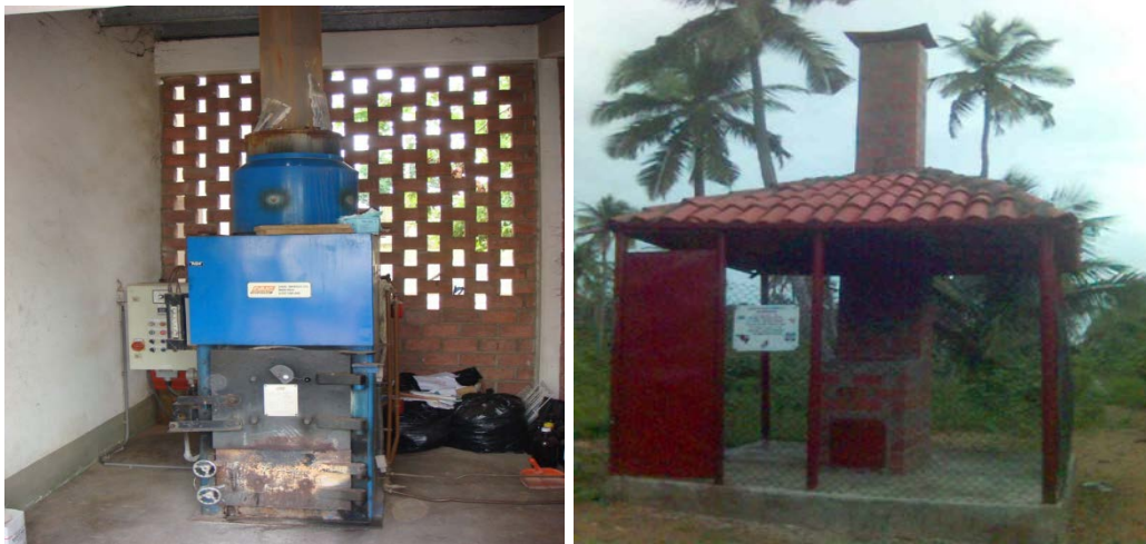
Figure 3. Examples of an Incinerator and a Waste Disposal Unit
