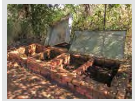
Two Tank System
