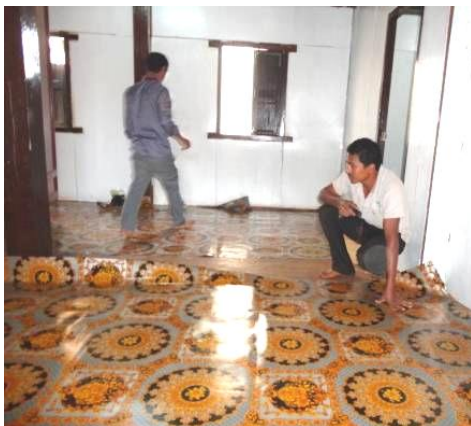
Refurbishment of the new MRDC office on the first floor of the ecotourism centre supported by WWF
