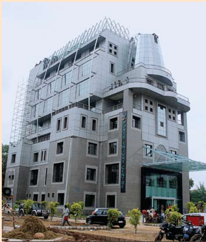
Asia's first Sports Injury Centre (SIC) at Safdarjung Hospital constructed in record time of one year in 2010
