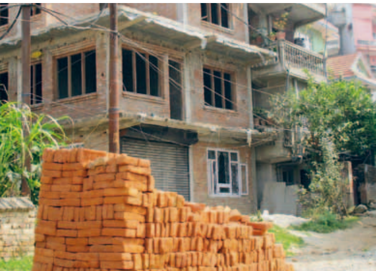
Photo8a: Poor quality bricks © UN-HABITAT
