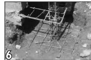
6 Extend column reinforcement with proper lap and proper foot to reinforcement pad in foundation
