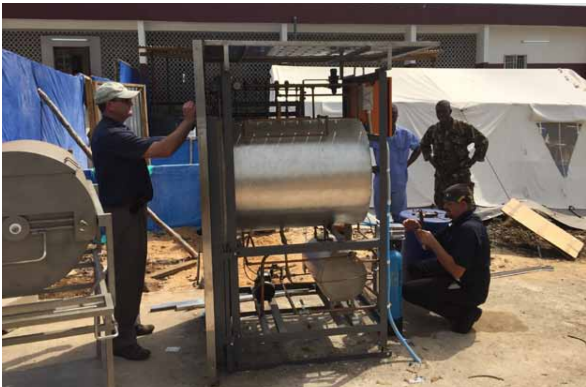
Autoclave being installed in Sierra Leone to treat medical waste. (Photo: UNDP)
