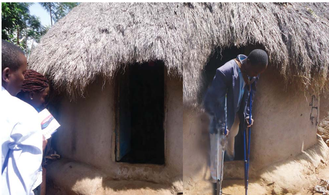
Lack of physical access is not only at public buildings but also within homesteads. One of the homesteads sampled during the monitoring
