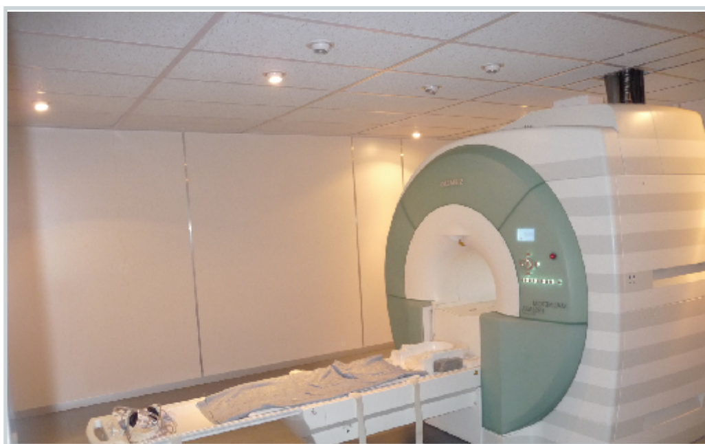
MRI equipment at Cancer Hospital
