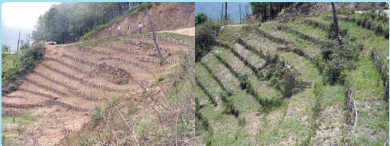
Figure 26: Newly constructed bench terraces on a slope (left) and the same terraces some years later (right)
