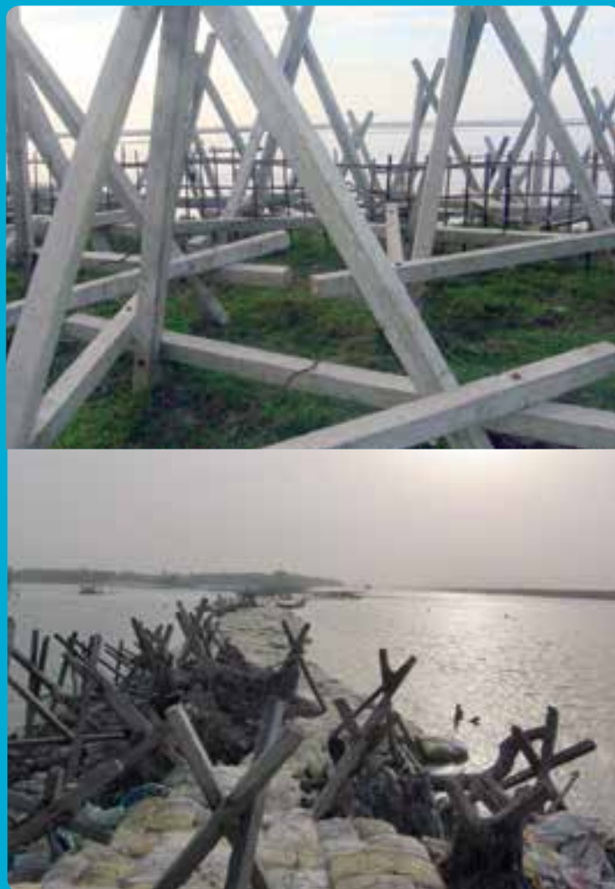
Figure 51: RCC porcupines along a river bank (top) and combined with sandbags to form a bar projecting into the Koshi river (bottom)
