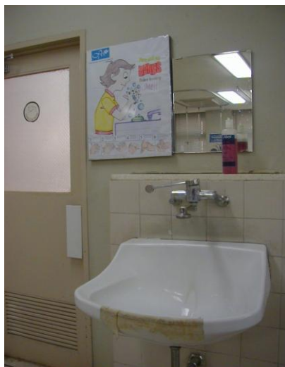
A hand washing reminder, but the sink is unsafe as it has a taped crack
