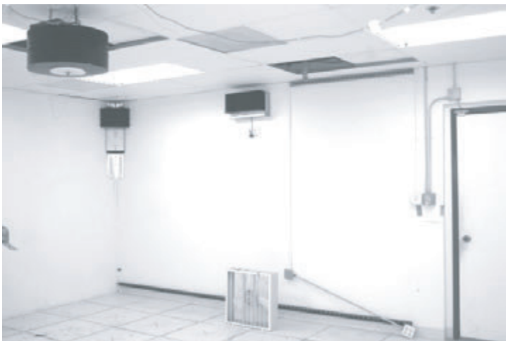
Corner wall and ceiling mounted UVGI fixtures
